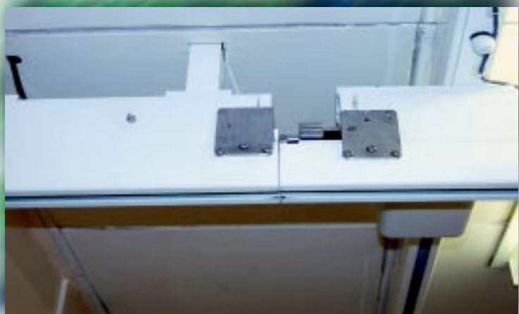
A simple connection with automatic engagement between track sections allows transfer to the Post Mortem Room
